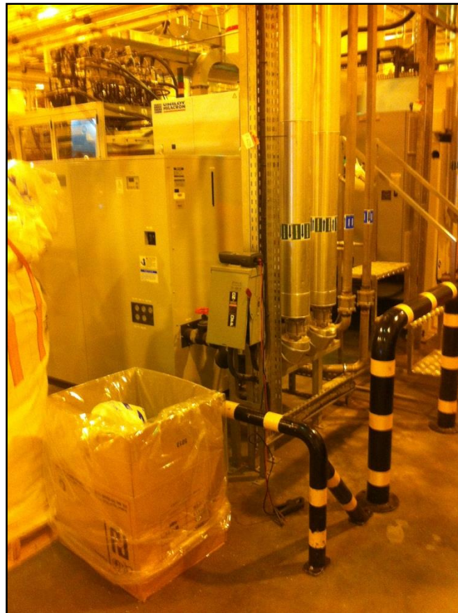
Picture 5: Inner photo from the Bottling Machine lines sector
