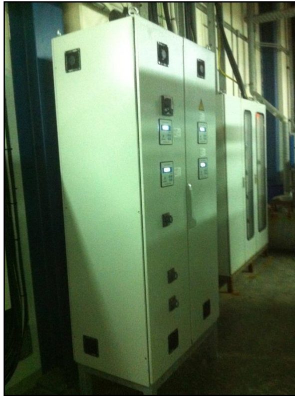
Picture 10: Four (4) different SEMAN DMCC's customized Low Voltage (LV) Variable Interventions, combined at a single enclosure installed at ALMARAI's electrical installations
