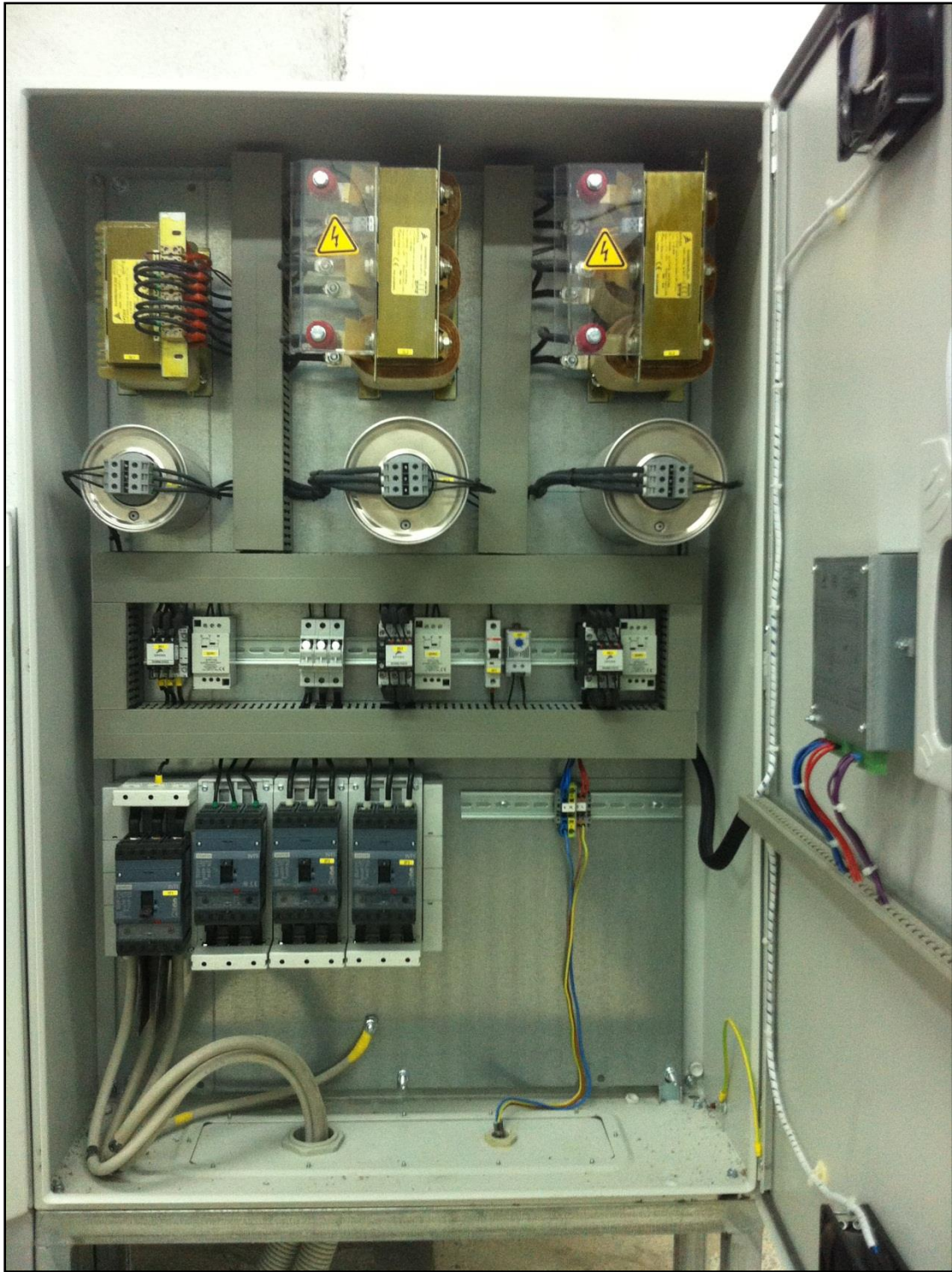
Picture 15 : SEMAN DMCC's customized LV Variable Intervention installed at ALMARAI's electrical installations – Detail of Inside view
