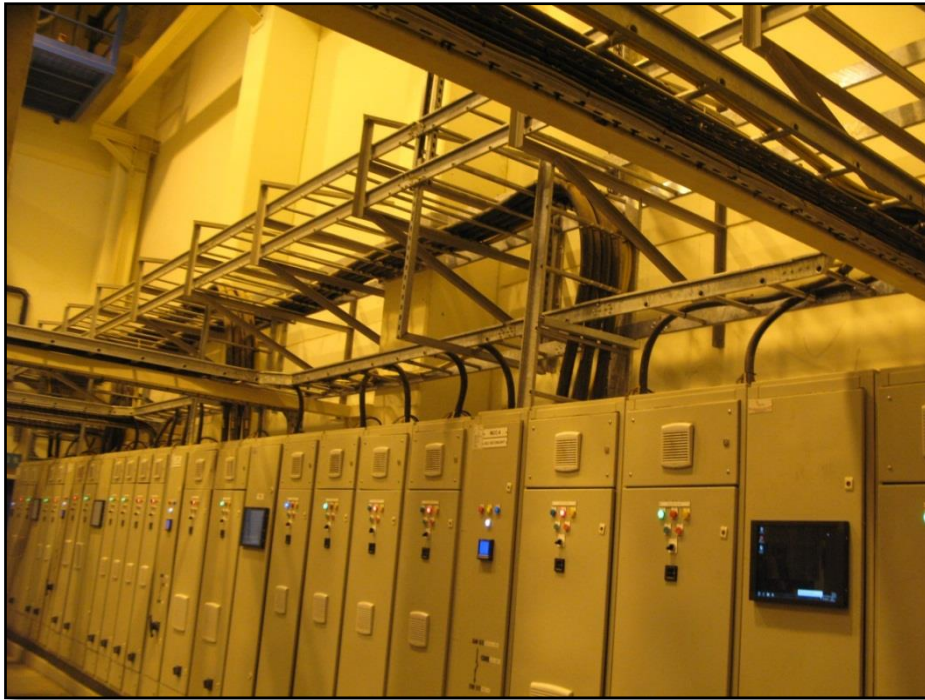
Picture 4: Compressors & Pumps distribution panel room
