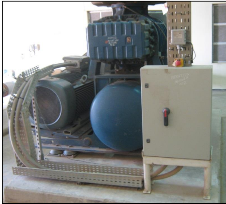
Picture 7: Measurements & recordings have been performed also in the core of the electrical installations next to the loads
