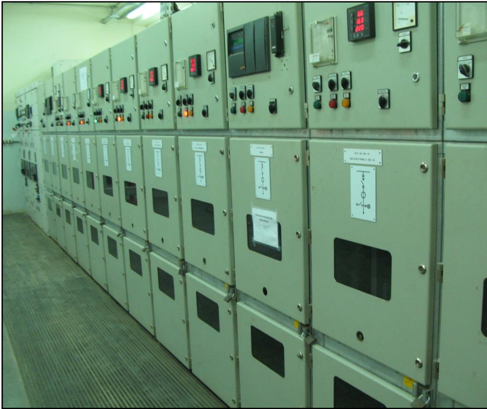
Picture 3: Medium Voltage Panels in one of the Main Electric Power Distribution Substations
