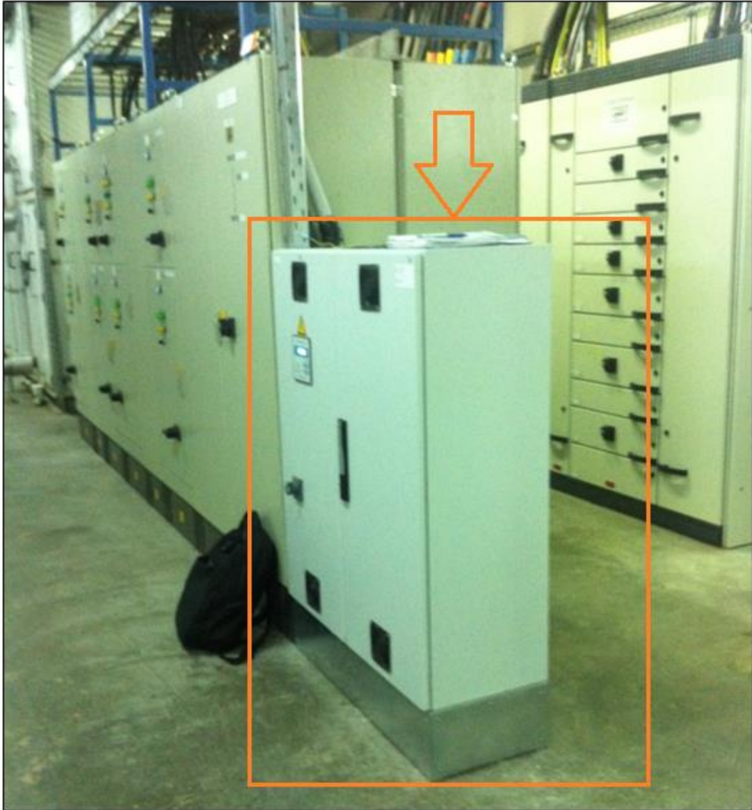
Picture 12 : Outside view of SEMAN DMCC's customized LV Intervention installed at ALMARAI's electrical installations
