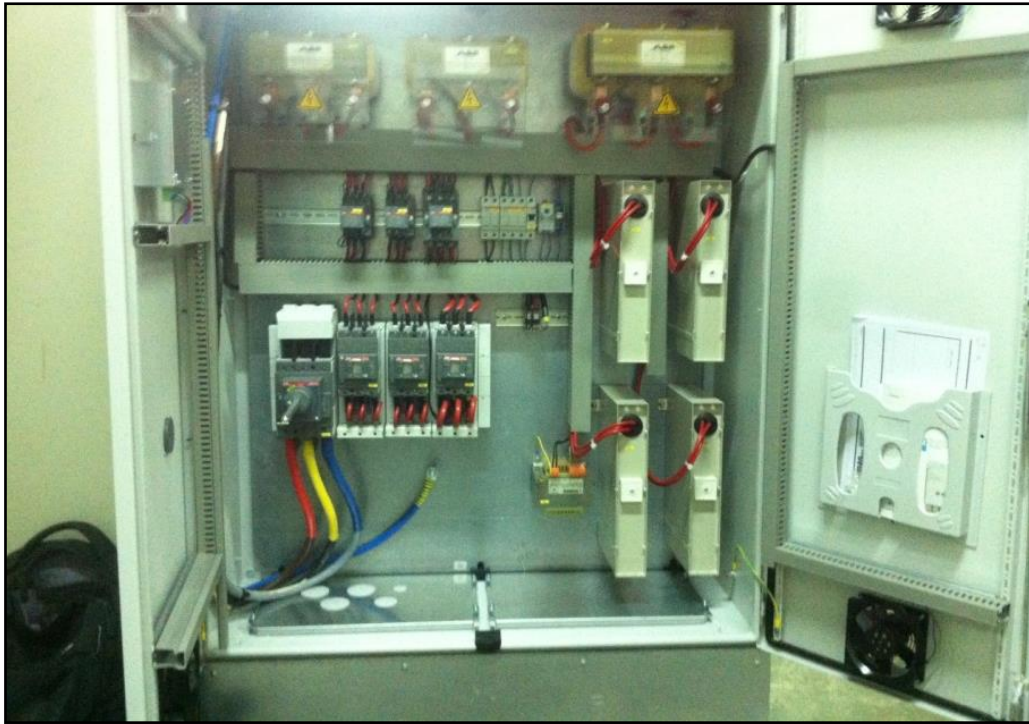
Picture 11 : Inside view of SEMAN DMCC's customized LV Variable Intervention installed at ALMARAI's electrical installations
