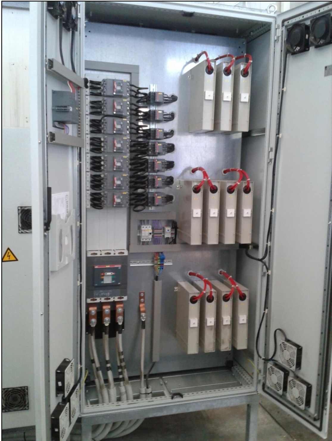
Picture 13: Inner side of SEMAN DMCC's customized LV Variable Intervention installed at ALMARAI's electrical installations
