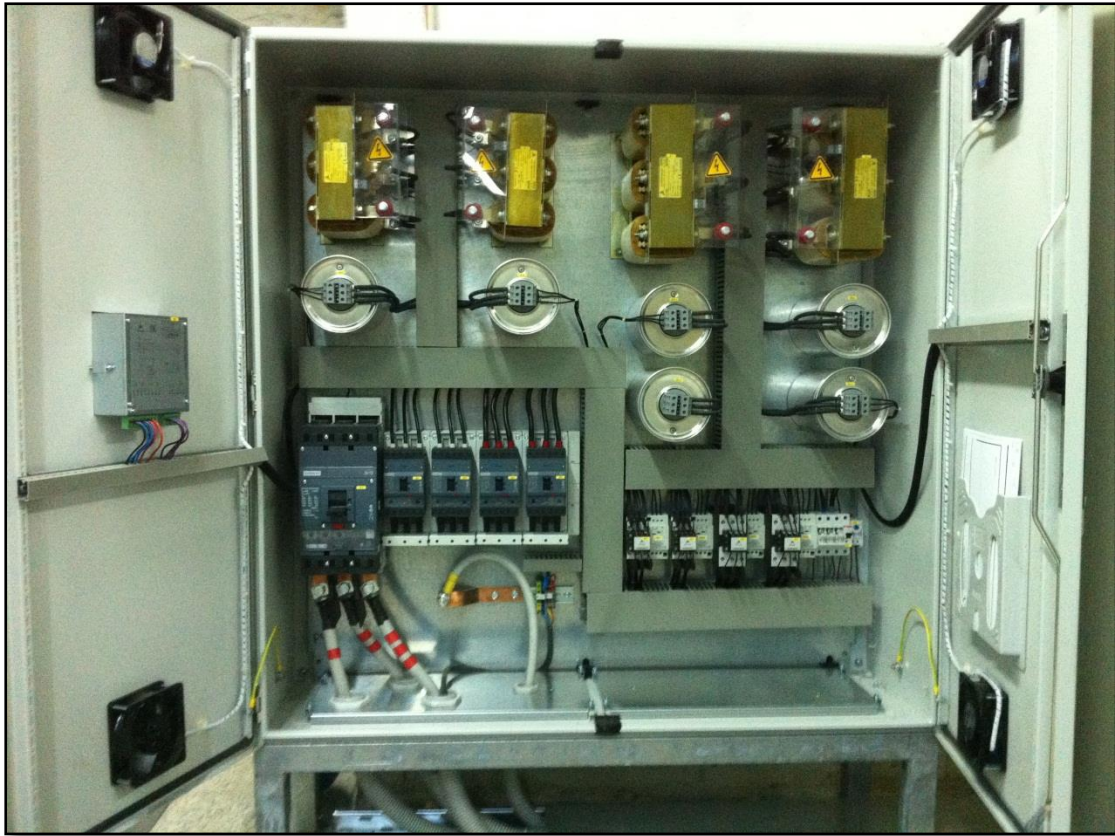
Picture 16: SEMAN DMCC's customized LV Variable Intervention installed at ALMARAI's electrical installations – Detail of Inside view
