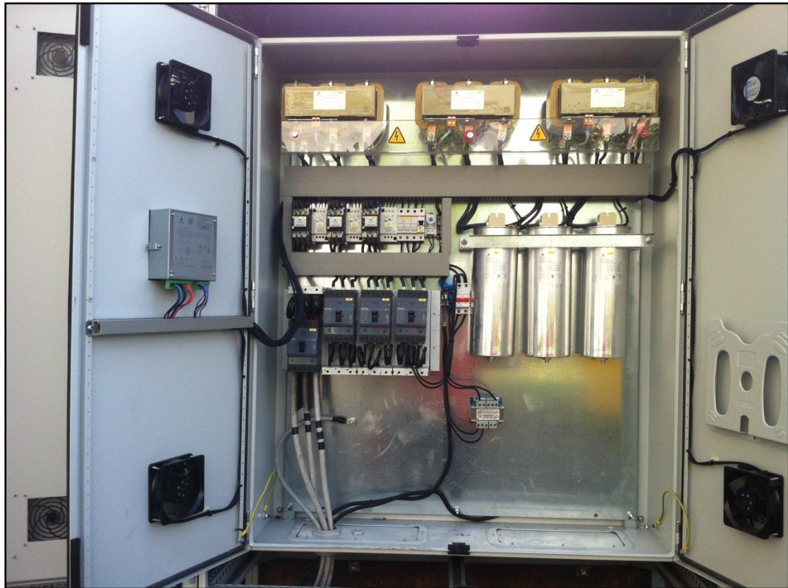
Picture 14: Inner side of SEMAN DMCC's customized LV Variable Anti-resonance Harmonic Filter, with adverse environmental conditions standing materials, installed at ALMARAI's electrical installations
