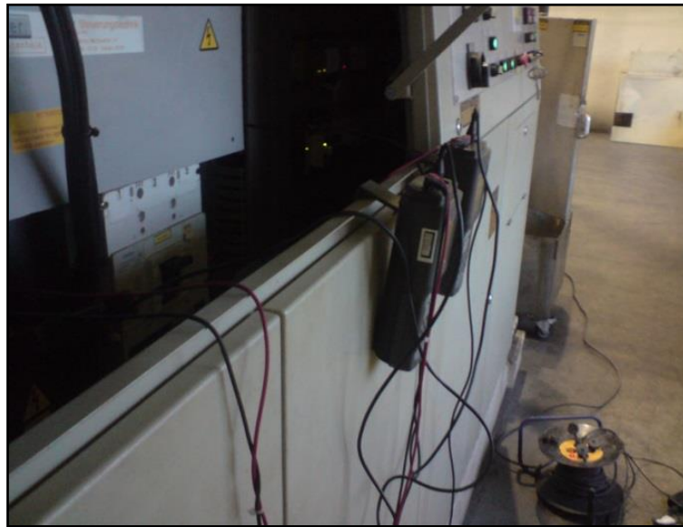
Picture 6: Power Quality Analyzers & Laptops were used for measurements and recordings
